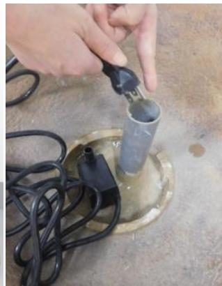
Pass the power cord from the pump down the cord pipe in the large bowl then down the pedestal.
