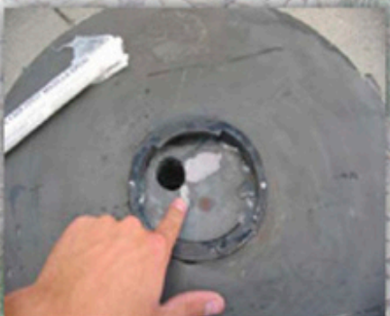
For this bowl, putty was applied in the crack and along the surface area.
