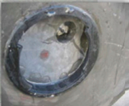
Locate leak in bowl. (In this scenario the leak is a small crack that has developed in the base)
